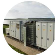
Grid stabilisation technology
