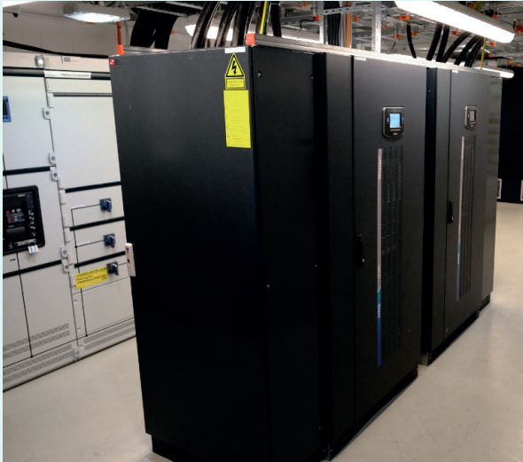
2 x 250 kW Master+ UPS
